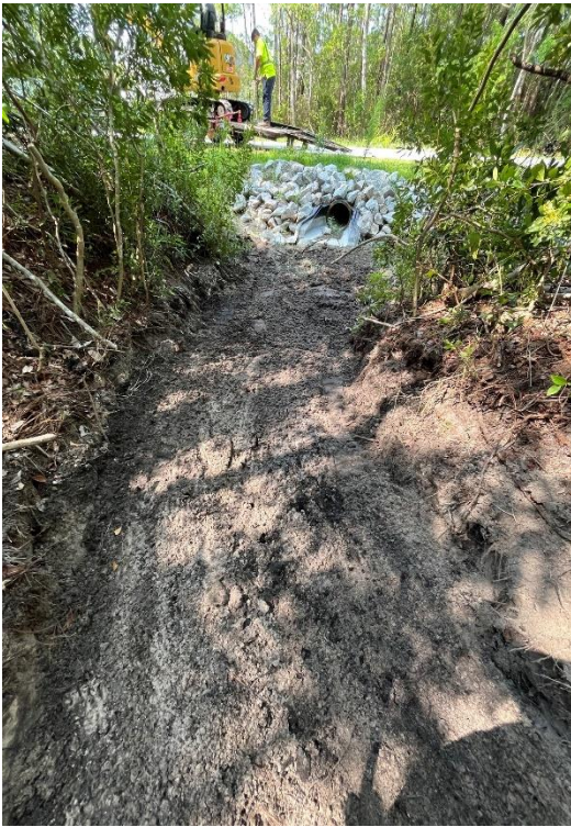
Filmore Road Discharge Outlet Protection
