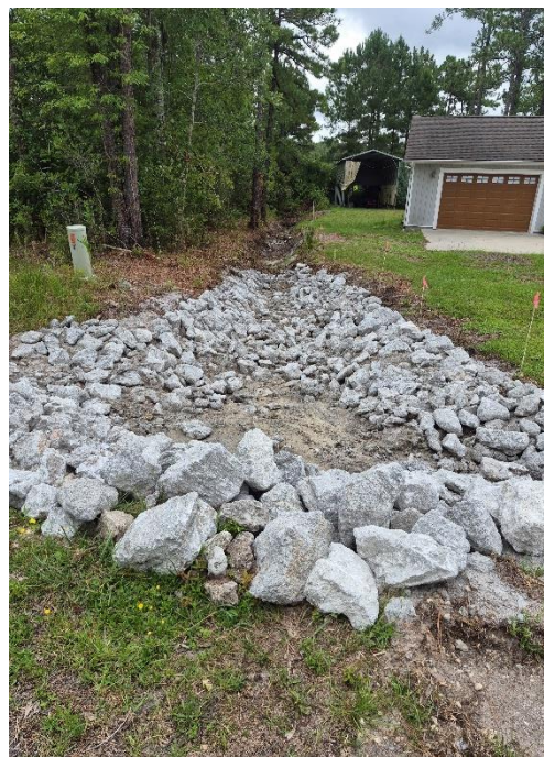
North Shore Drive Rip-Rap Channel Protection
