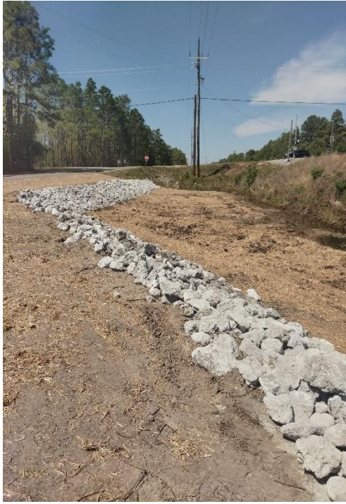
Fifty Lakes Drive Basin Rip-Rap Slope Protection
