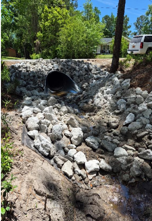
Windemere Pipe Upgrade Downstream Flared End Section and Rip-Rap Protection
