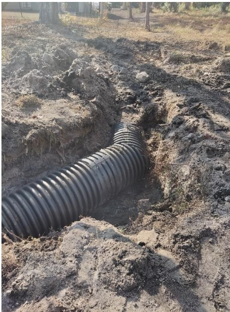
Pipe Culvert 45 degree Bend
