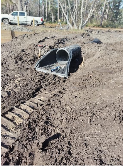
Pipe Discharge w/Flared End Section
