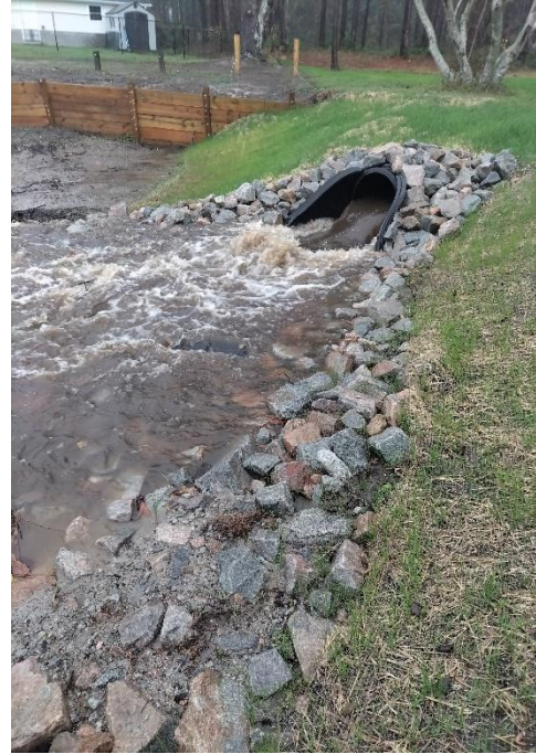
Pine Lake and Miller Pipe Discharge
