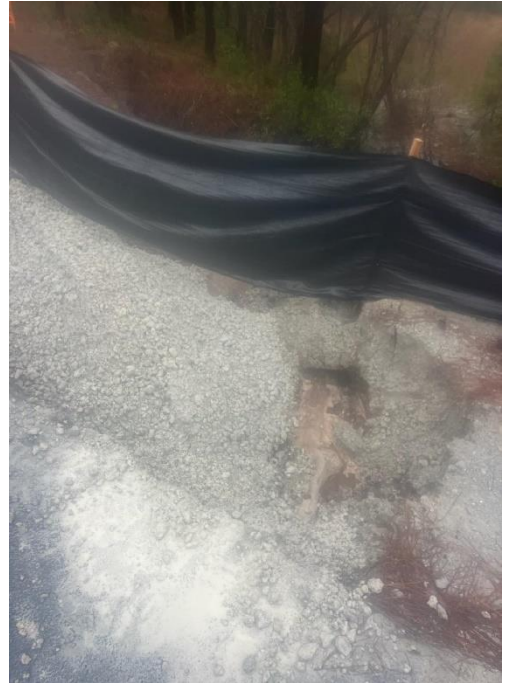
South Shore Drive Street Washout
